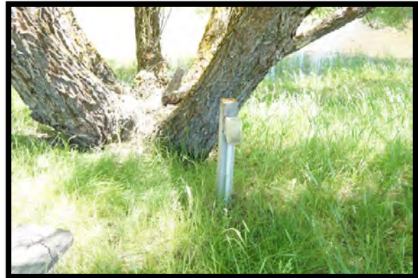
Power Outlet at River Frontage
