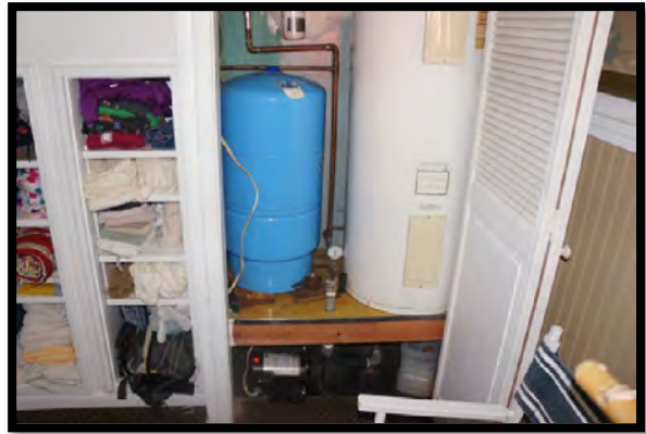
Closet & Water Heater
