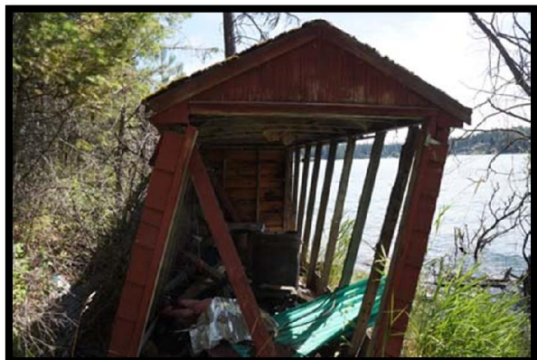
Depreciated Storage Building near Lake
