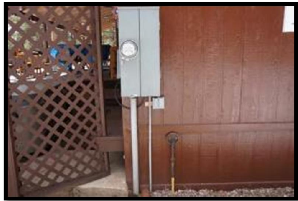
Electrical Meter on East Side of Residence
