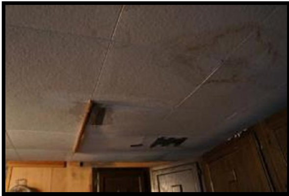
Water Damage on Ceiling
