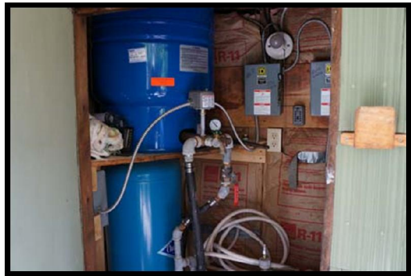
Well Pump Equipment
