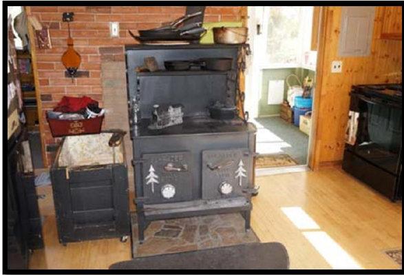
Woodstove in Kitchen
