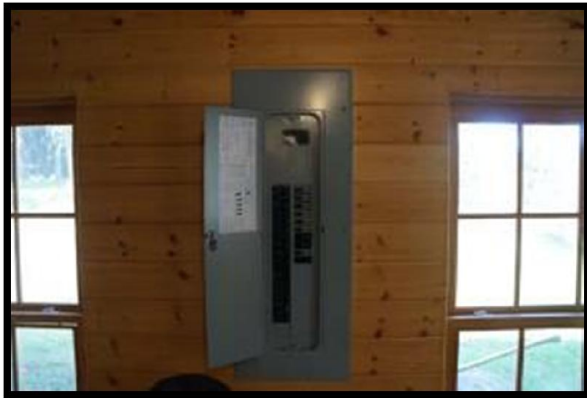
New Electrical Panel
