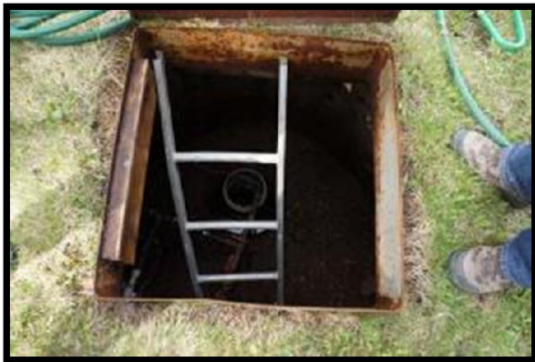
Water Pump Enclosure
