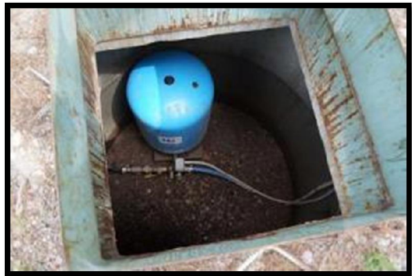
Well Pump Enclosure and Water Tank
