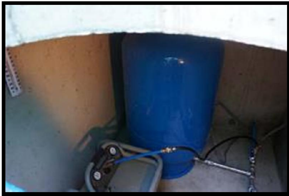
Water Tank and Pump Equipment
