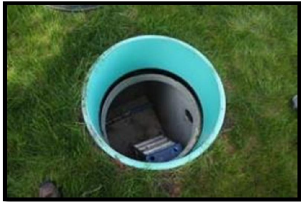
Water System Vault
